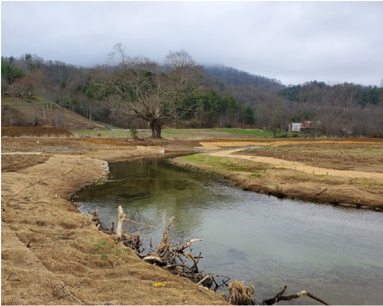
Dutch Creek stream restoration project after instream construction and just before planting the riparian buffer.
