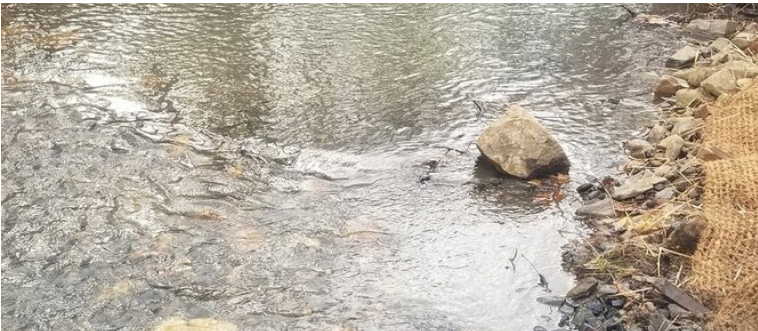
A view of the in-stream structures installed on Call Creek. The in-stream structures will improve aquatic habitat.
