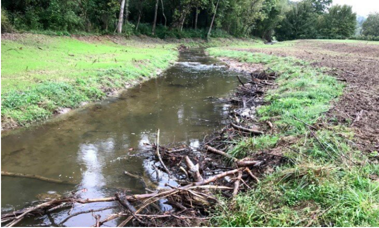
This restoration project is located on a stream reach at the confluence of Garringer and Little Brasstown Creek.
