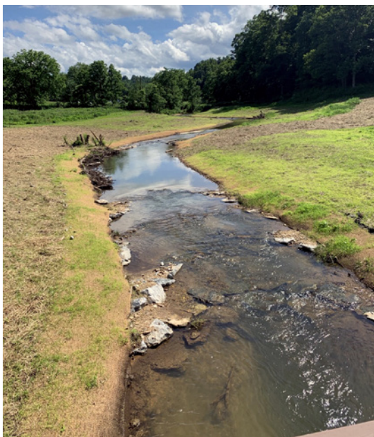
A restored reach of Reedy Patch Creek immedi- ately following in-stream con- struction.
