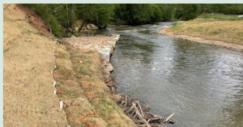
RI is working with Surry County to address streams damaged by large storm events. The work is being completed under NRCS's Emergency Watershed Protection Program (EWP).
