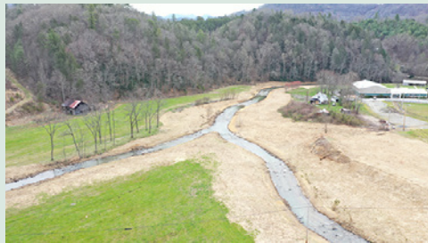
Ivy Creek project - The confluence of California, Paint Fork, and Little Ivy creeks in Mars Hill, immediately after undergoing stream restoration.
