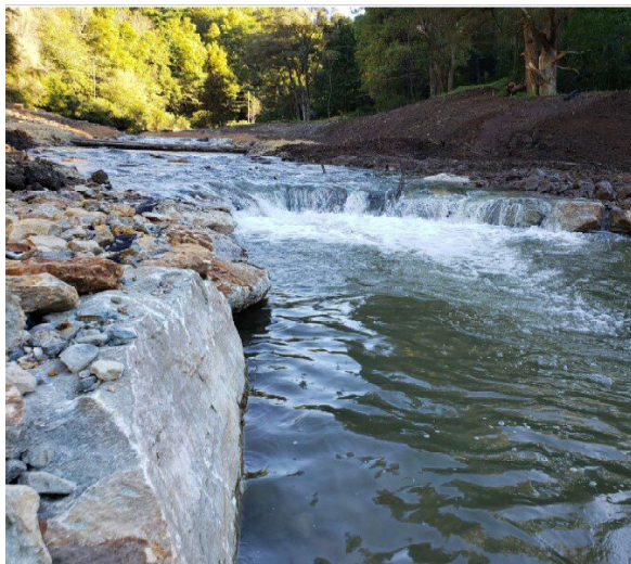
A j-hook vane constructed upstream of the former dam site on Payne Branch.
