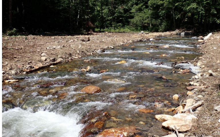
Instream structures constructed to stabilize Catheys Creek above the City of Brevard Water Treatment Plant.
