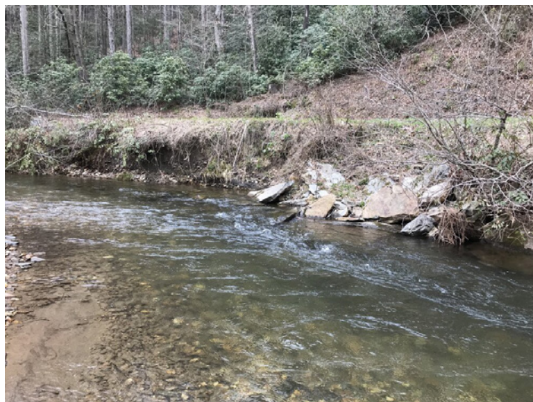
BEFORE: Prior to restoration, Catheys Creeks streambanks were eroding causing the adjacent road to be unstable as well.
