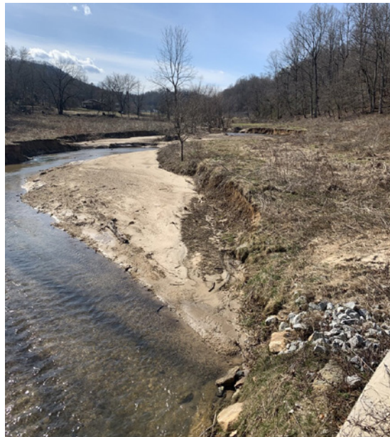
BEFORE: Reedy Patch Creek's eroding streambanks prior to resto- ration.
