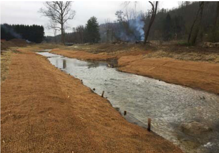
The project team planted a riparian buffer on Shaw Creek after instream construction is complete. The buffer is enhanced with Elderberry that the Farm will use for medicinal purposes.
