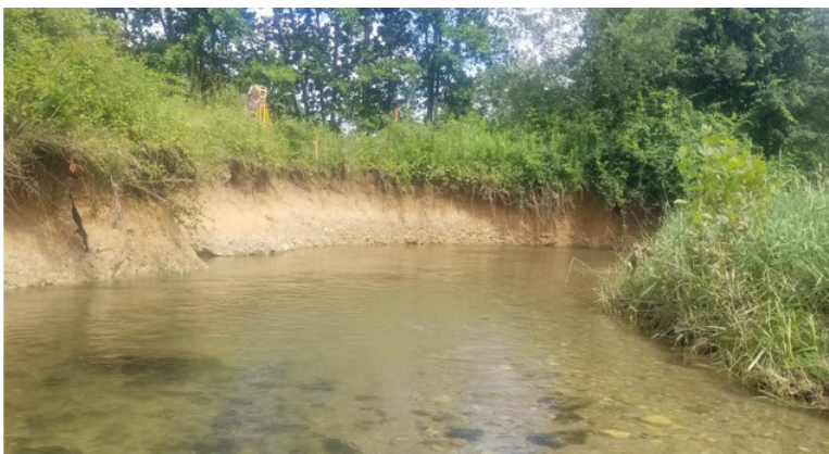
BEFORE: Dutch Creek was actively migrating and lacked proper dimension, pattern, and profile, as well as riparian buffer and aquatic habitat.
