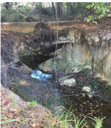
A number of agriculture ponds in Eastern North Carolina were damaged by hurricanes in 2016. This pond's dam was breached during the storms.
