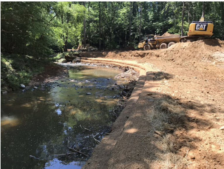
The Grassy Creek at Pilot Mountain State Park during instream construction of the restoration project.
