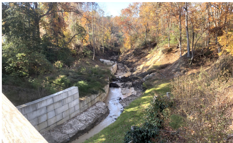
BEFORE: The creek was severely eroding and putting infrastructure at risk. High water from major hurricanes damaged a footbridge that connected the main campus to the University's PGA Golf Program and Center.
