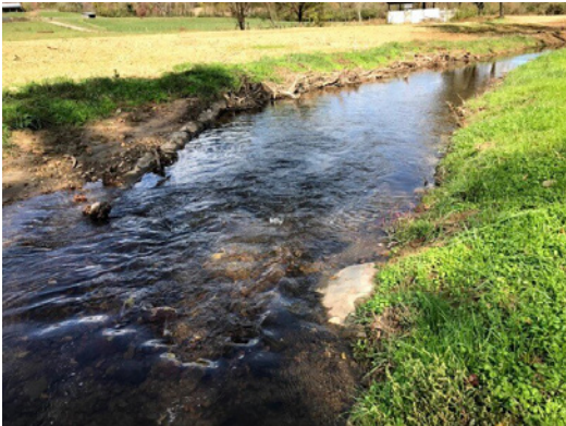
The Little Brasstown project employed several Natural Channel Design techniques. The project team realigned the channel and excavated the floodplain. They also installed log j-hook vanes, toe wood revetments, and cobble riffles.
