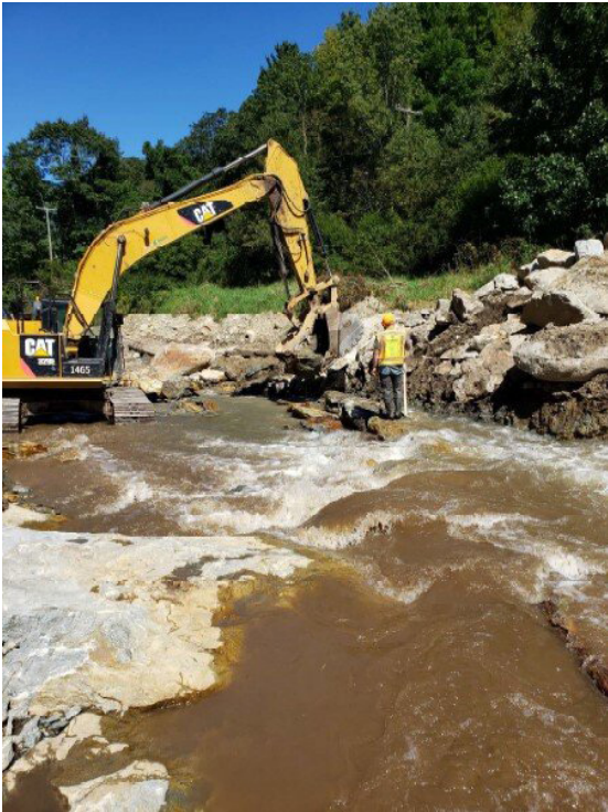
Construction of a cross vane on Payne Branch as part of the restoration project.
