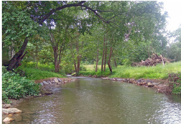
Instream structures just after construction on the Little Crabtree Creek restoration project.
