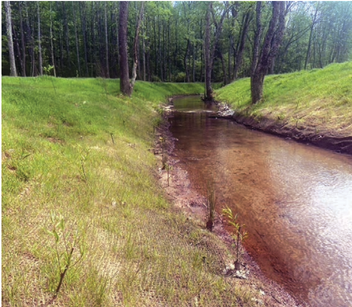
This photo is looking upstream of Pound Mill Creek post-construction and prior to riparian buffer planting.
