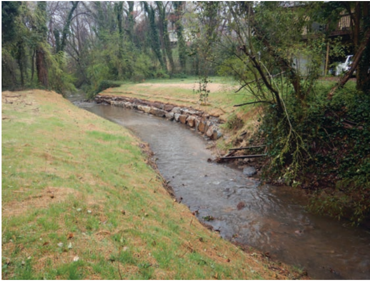
A completed EWP project along a reach of stream in Forsyth County, North Carolina. This stream was impacted by Hurricanes Florence and Michael in 2018.
