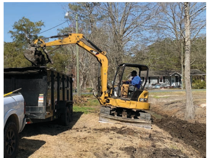
Sediment removal on a stream damaged by a significant storm event in Hoke County, North Carolina
