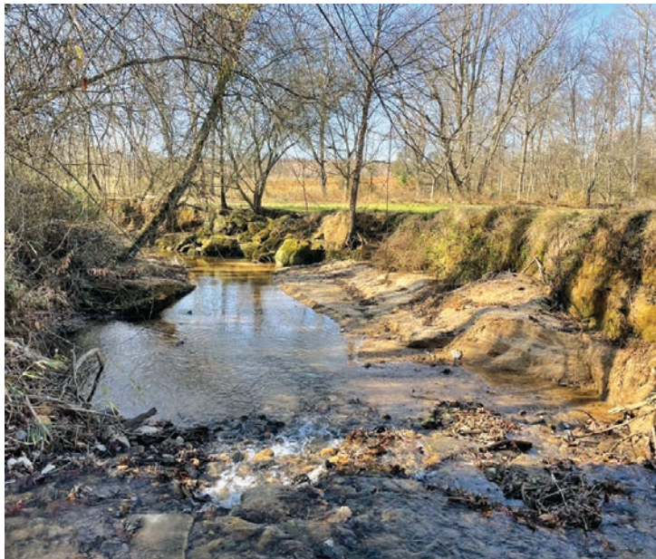
Prior to project implementation, Pounding Mill Creek and Knob Creek streambanks were steep and unstable.
