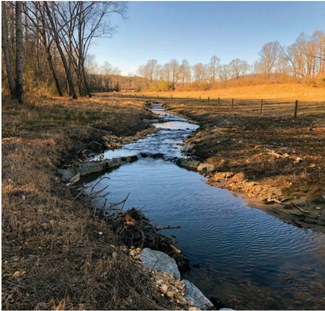
Hodges Creek post-construction showing in-stream structures and prior to riparian buffer planting.
