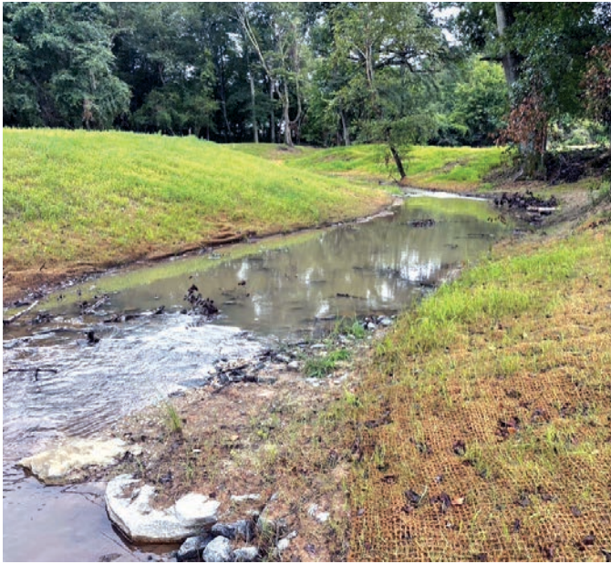
This photo looks upstream of UT to Second Broad post-construction and prior to riparian buffer planting.
