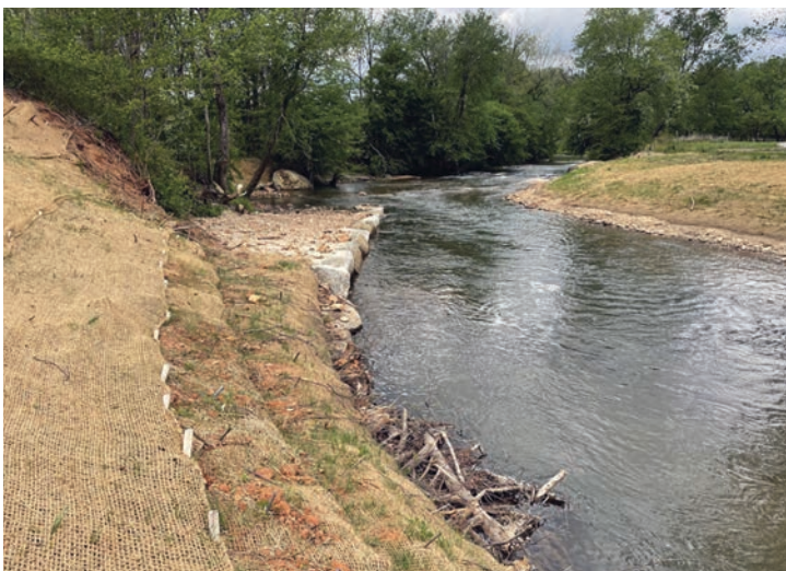
Resource Institute implemented a stream restoration project as part of an EWP project in Surry County, North Carolina.
